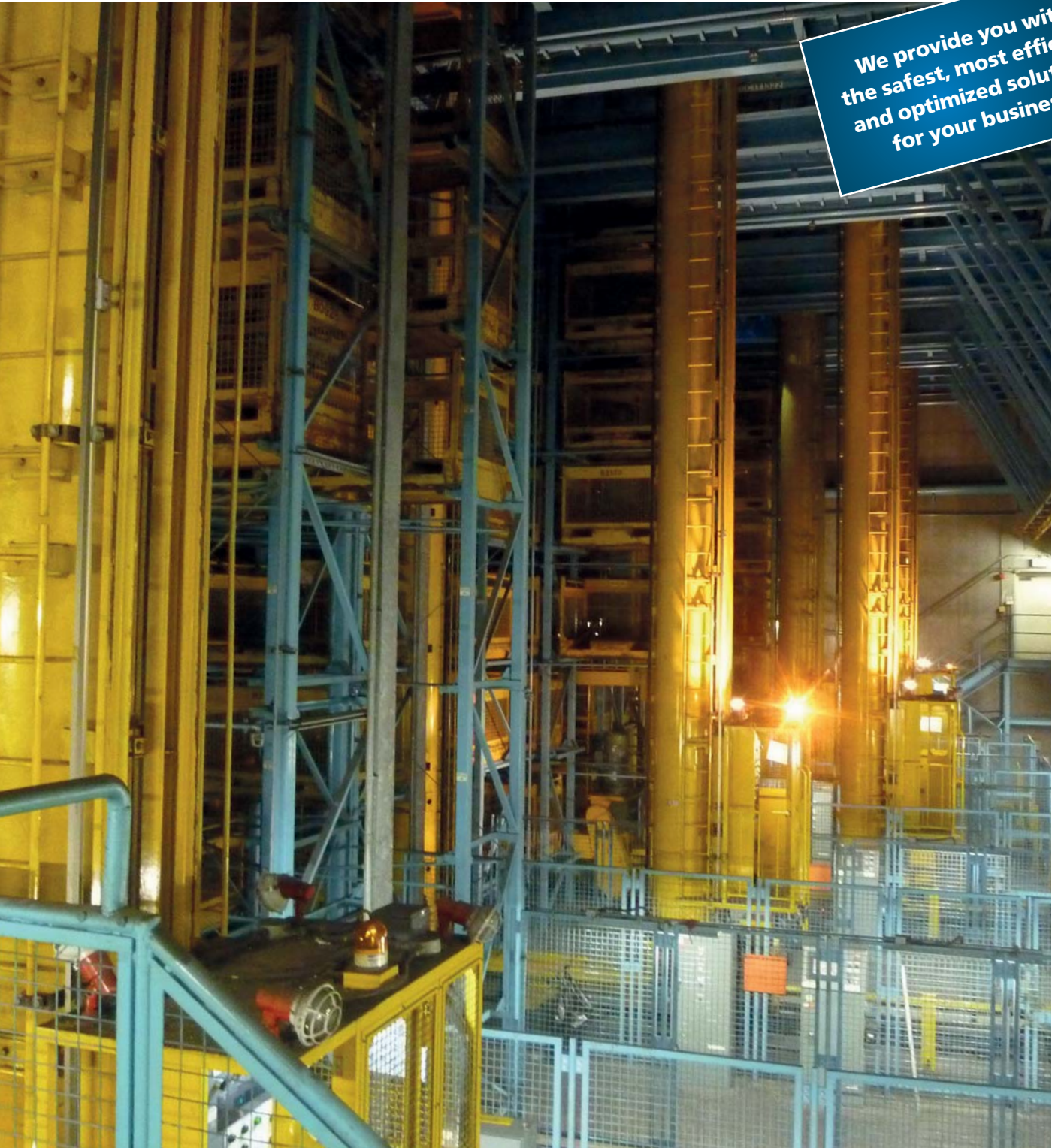
Picture on Front Page: Hong Kong Air Cargo Terminals Ltd. (Hactl), Box Storage System (BSS)
